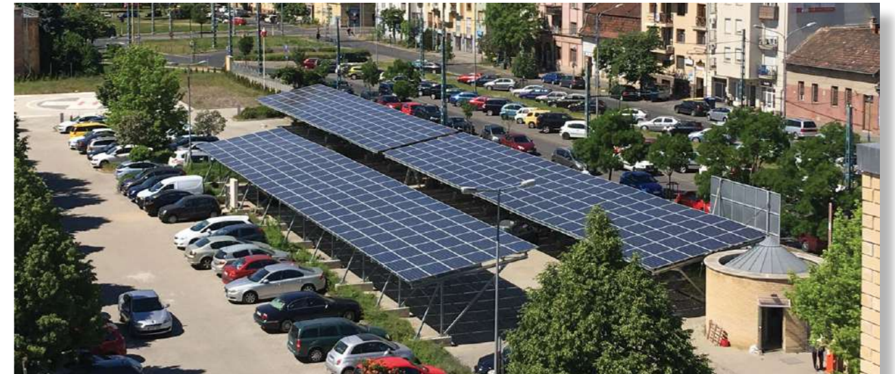
Budapest, Uzsoki street - 424 kWp
