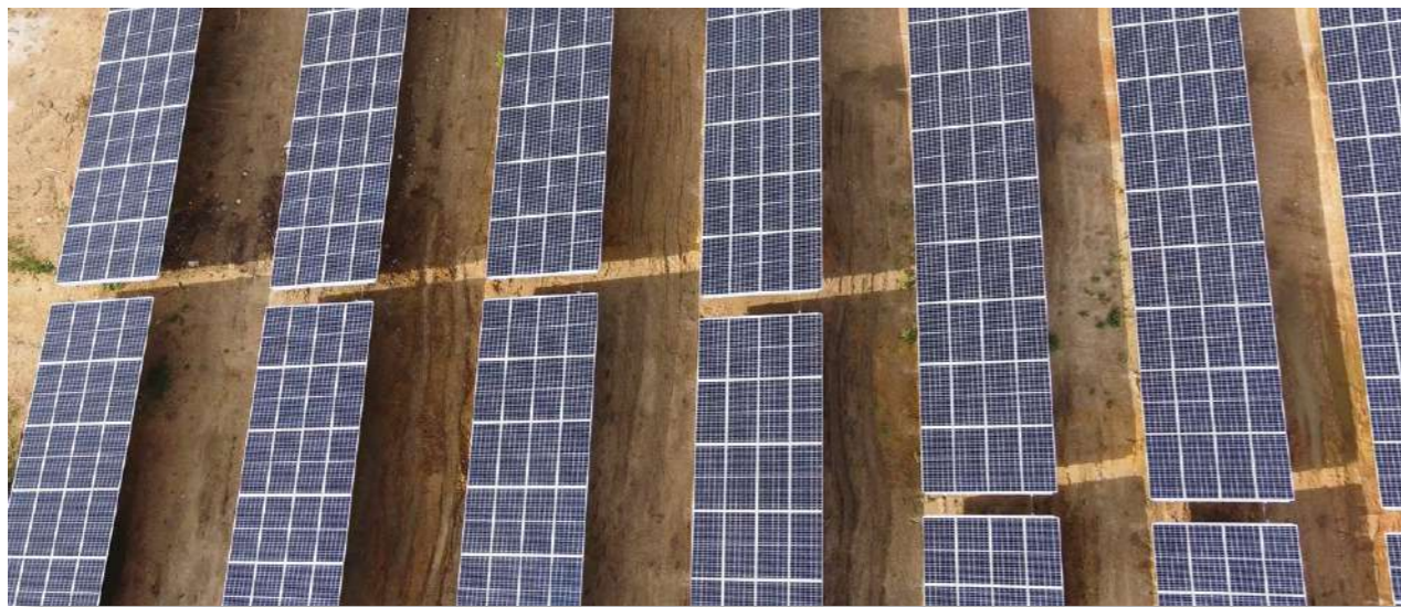
Nyírad (Own power plant) - 1 MWp
