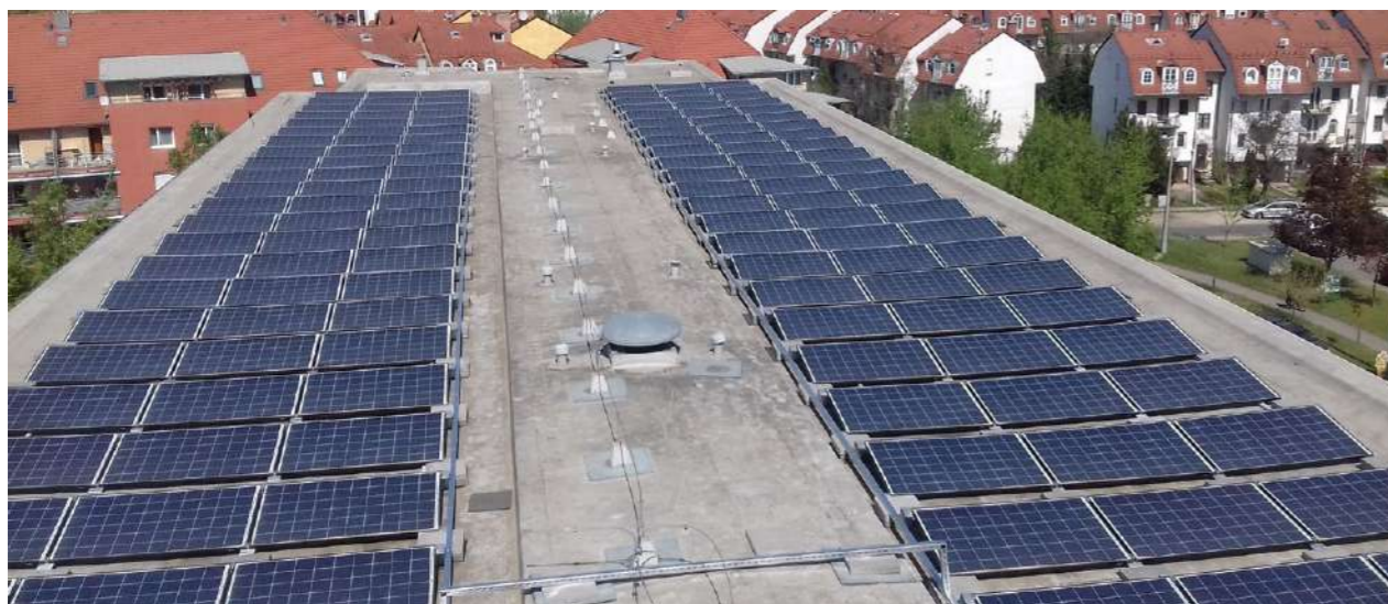
Dunakeszi Police Headquarters - 51.87 kWp
